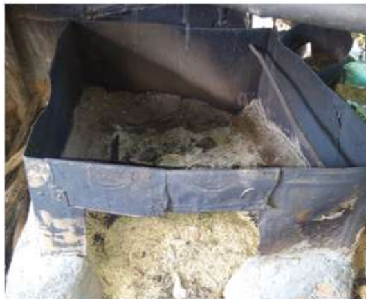
Photo Plate 7: Furnace chamber
